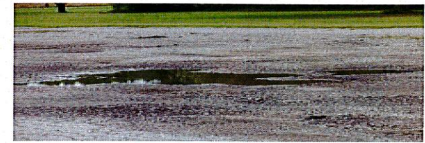
Pools of standing water form after rainfall.
