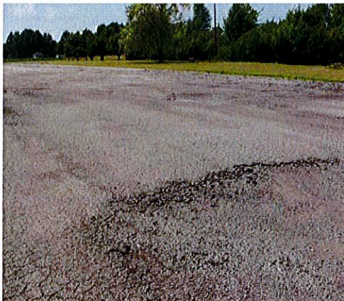
The crumbling pavement and the bumpy potholes make driving into the Shrine parking lot an unhappy adventure.
