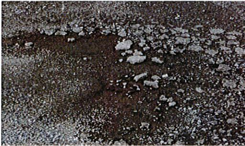
The deterioration of the parking lot is quite noticeable.
