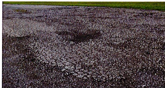
The crumbling of the pavement is quickened by Ohio's harsh winter storms.
